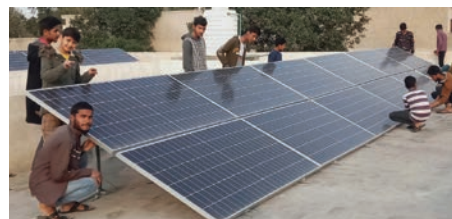
The new solar panels have made a huge difference in the lives of boys at the Pakistani home.
